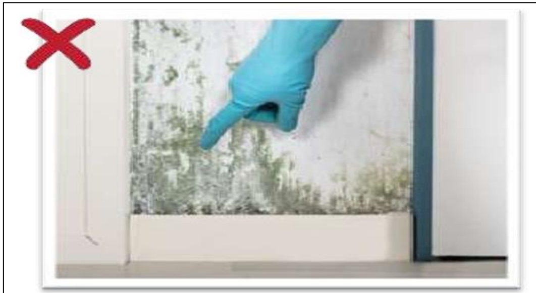
Fig. 29: Fungal growth (moss) on a wall
