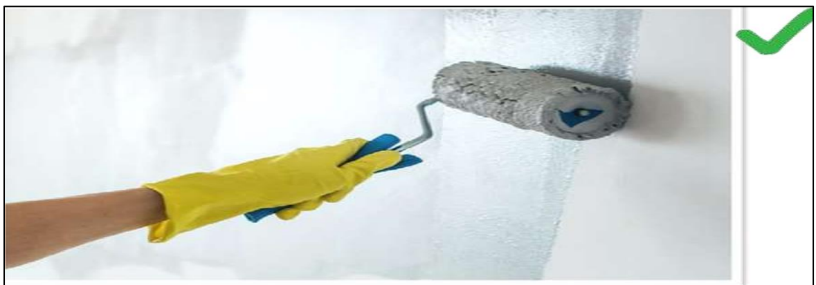
Fig. 28: Example of smooth, impervious wall and floor surfaces
