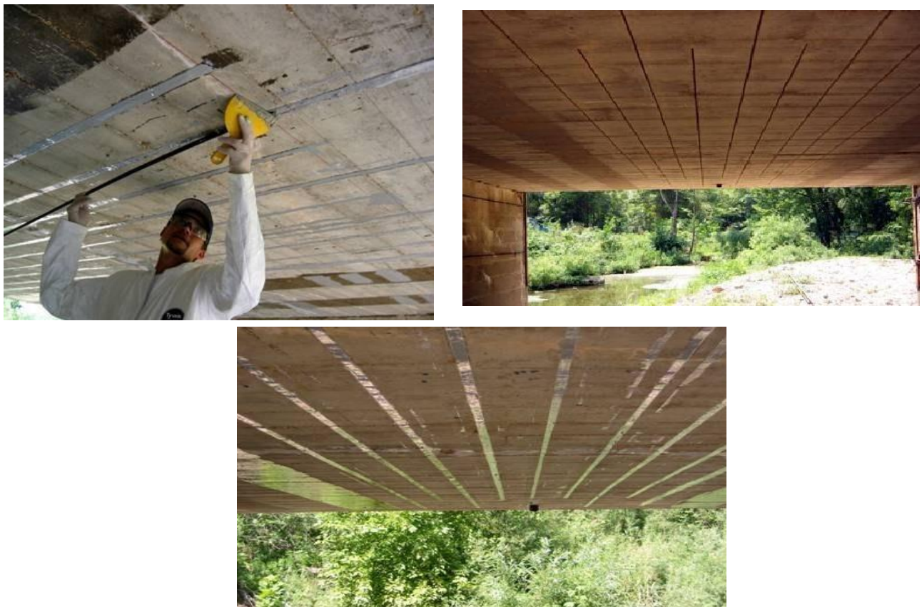
Figure 1.7 Main stages of the NSM strengthening: a) Grooving; b) Adhesive and FRP placement; c) Strengthened member [30]
