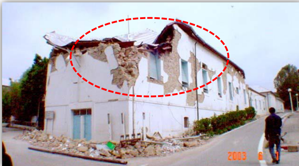
Figure 45: Effondrement total de l'hôpital de Thénia. (Sources : Earthquake Engineering Research Institute (EERI 2003))
