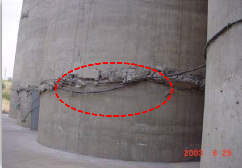
Figure 53: Endommagement des silos de la commune de Corso (Source : Rapport Japan Association of Earthquake Engineering (JAEE) et al., 2004)
